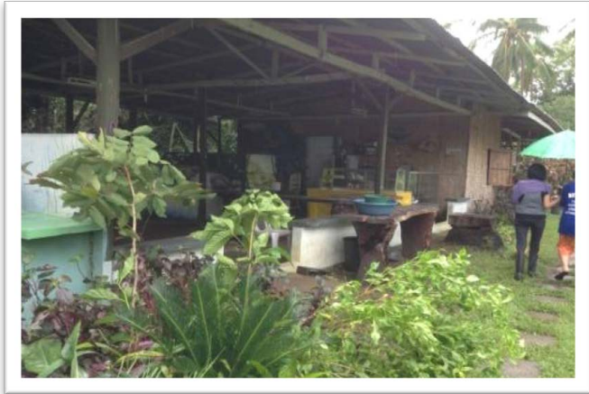
The mini-canteen and serving area after Typhoon Glenda.
